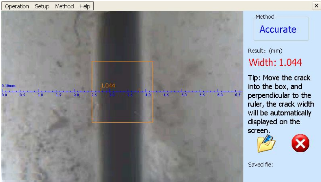
Figure 11 Saved Crack Image
